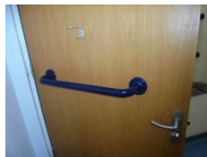
Door opens inwards rather than outwards
