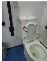
Emergency alarm cord too short
